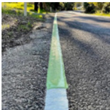
Figure 6. marking with green glow paint - photoluminescent/ glow in the dark road & line marking. Source: author's contribution.
