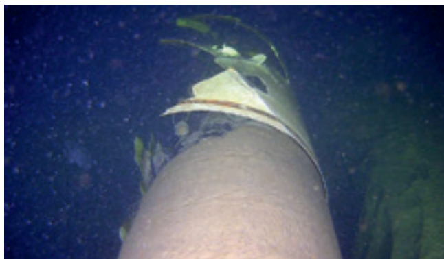
Fig. 3. The damaged offshore Balticconnector gas pipeline. Source: [8]
